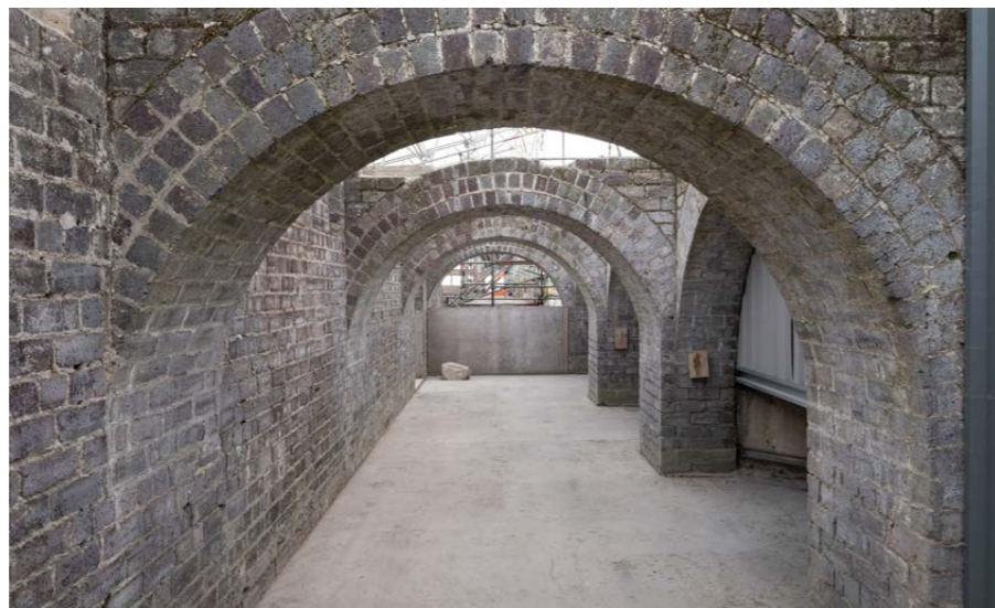
Image top / Ground floor, Reid Building Image right / Loggia, Mackintosh Building May 2024
